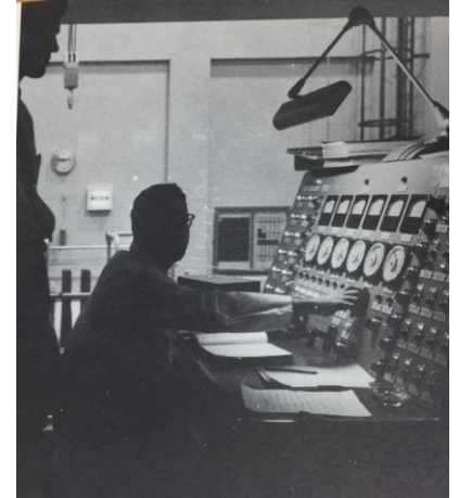
Figure 4. Photograph of a reactor operator at the FNR control panel
